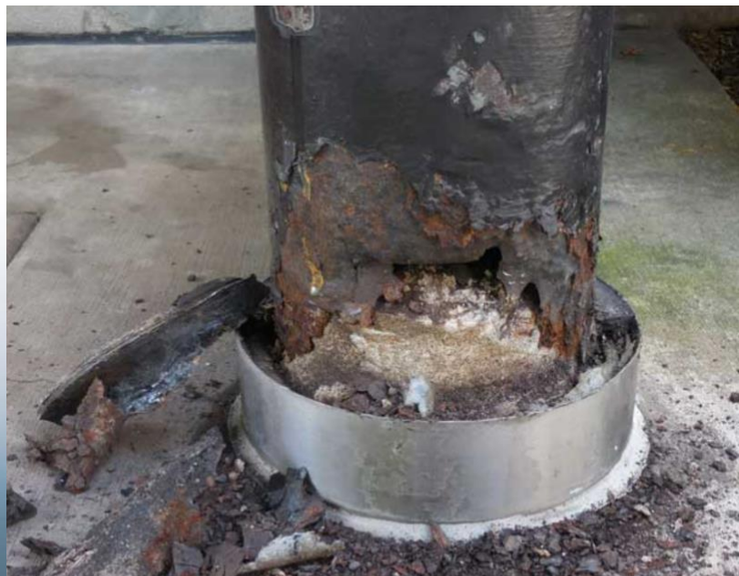
Below rusted through column
