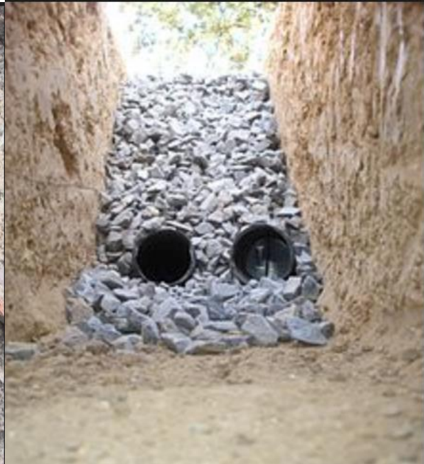
Curtain/French drains are 10 to 15 feet deep, a distance from the house foundation and generally wraps around the house to shed water away.
