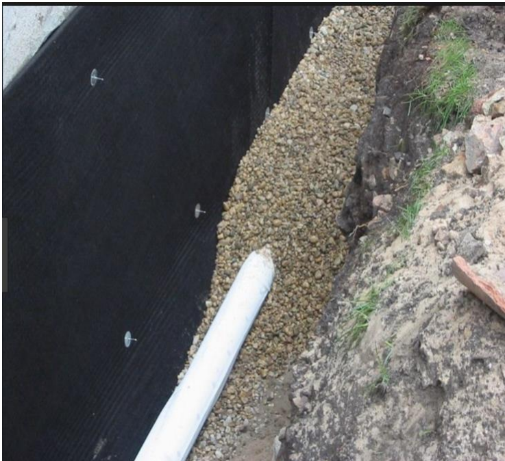
The Tile/Footing drain is installed during initial construction of the home at the base of the foundation footing.
