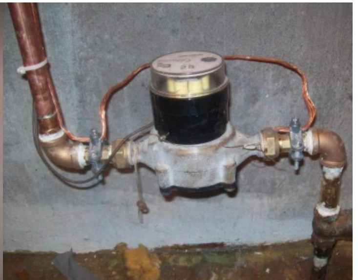
Bonding wire over a water meter.
