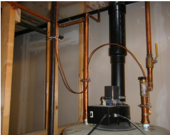
Bonding wire from cold water to hot water pipe and to gas line above a hot water heater.
